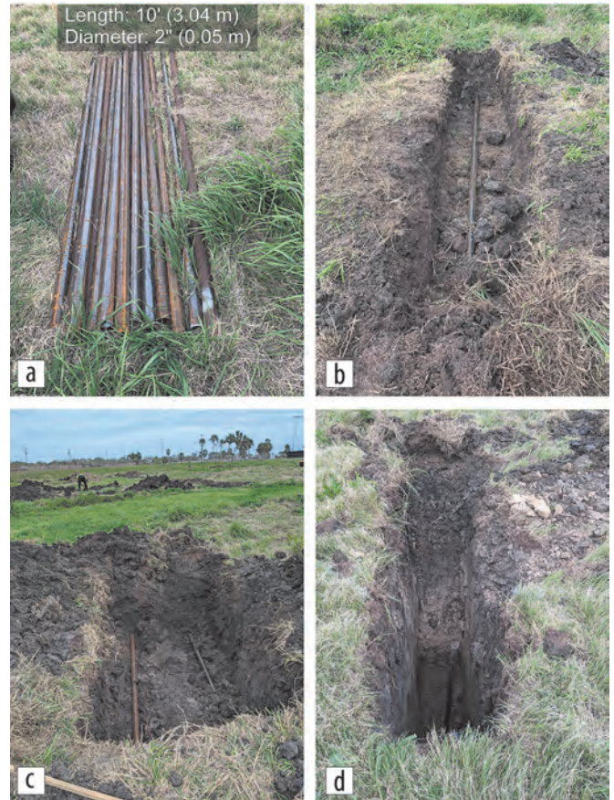
Figure 10. (a) Types and dimensions of steel pipes installed within the GTS. Also shown are (b) single horizontal, (c) double 1 m apart, and (d) vertical steel pipes.
